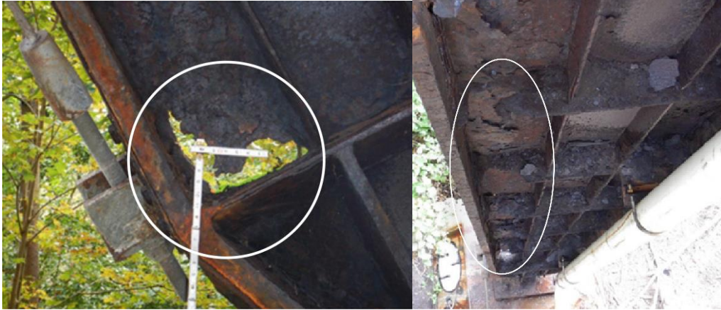
Figure 29. Corrosion of inside face of southwest leg (B1R). (Source: 2021 inspection report)
