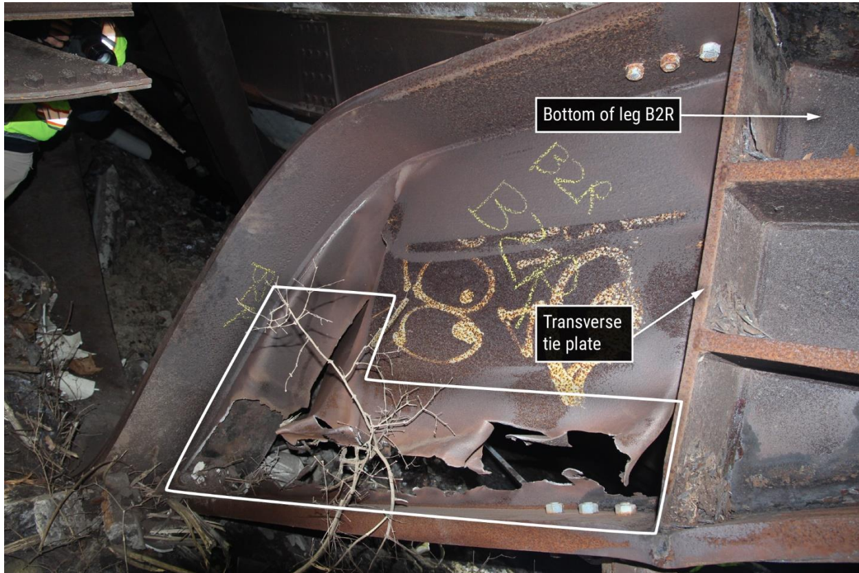
Figure 21. North-northwest-looking view of southeast leg (B2R) showing secondary fracture of the web, outlined in white.
