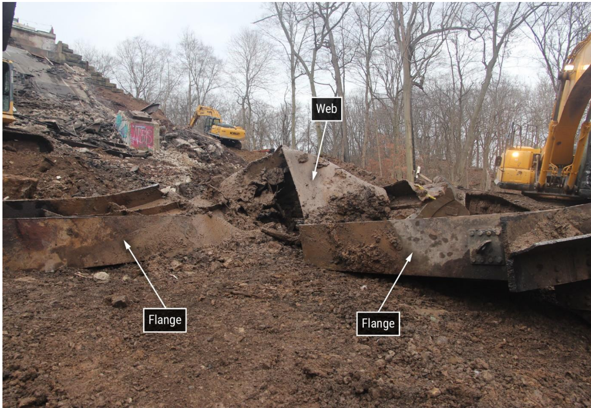
Figure 18. Northwest-looking view of northwest leg (B1L) after excavation, showing that portions of the flanges on both sides were no longer connected to the web.
