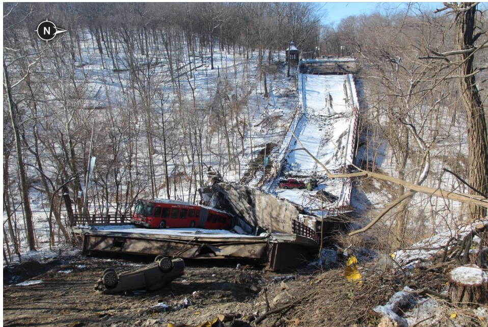
Figure 1. West-looking view of collapsed Fern Hollow Bridge.
