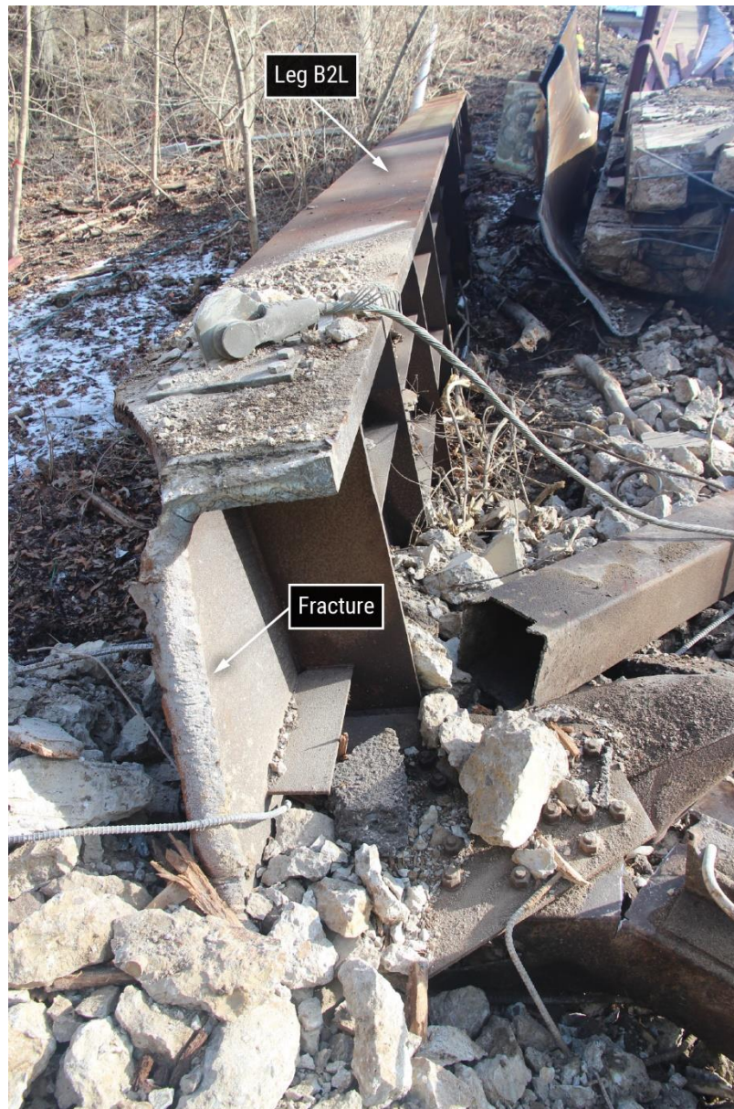
Figure 20. East-looking view of northeast leg (B2L) showing that the leg was intact below the fracture between the end plate and the top of the leg (the end plate is not visible in the photograph).
