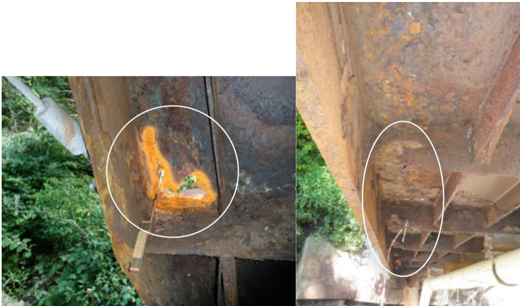
Figure 28. Corrosion of inside face of southwest leg (B1R). (Source: 2013 inspection report)
