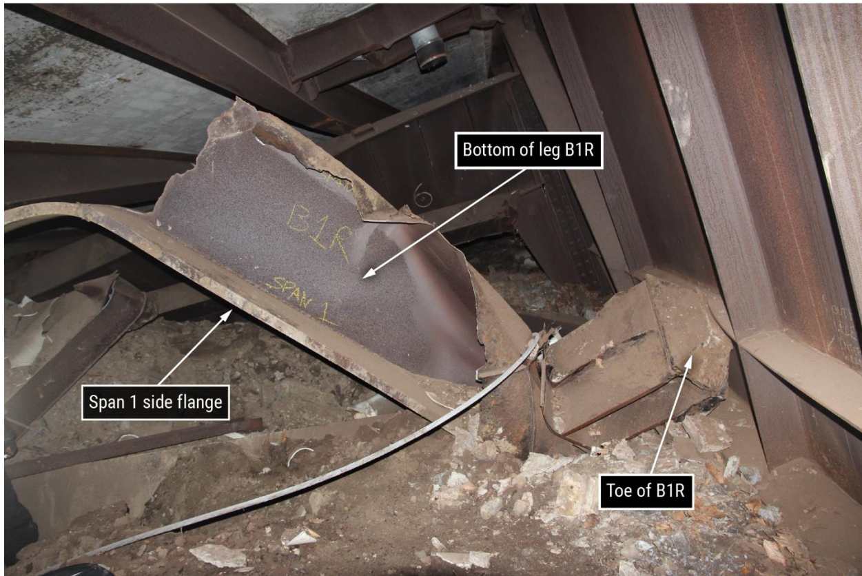
Figure 23. East-looking view of lower portion of southwest leg (B1R) underneath the collapsed structure.
