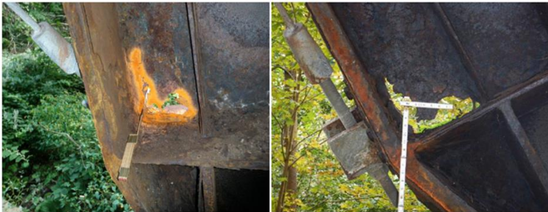
Figure 37. Corrosion damage including areas of 100% section loss on southwest leg (B1R) in panel 1 above the transverse tie plate. (Source: 2013 inspection report [left photograph]; 2021 inspection report [right photograph])
