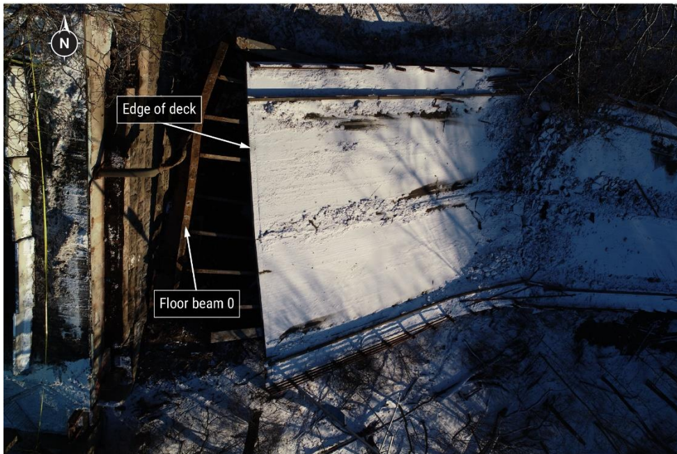
Figure 14. Overhead view of west (near) side abutment and bridge deck showing deck displacement east and south.
