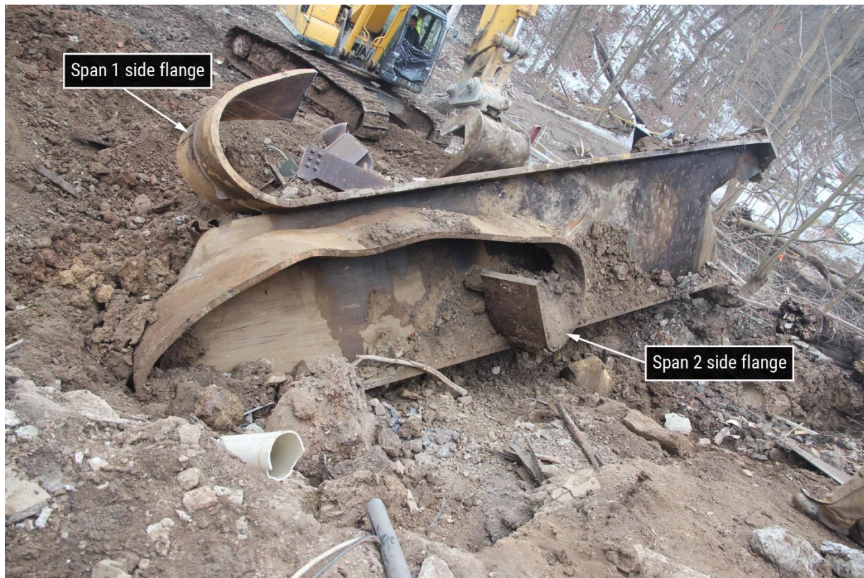
Figure 25. Southeast-looking view of upper portion of southwest leg (B1R) showing partial separation of span 1 side flange and significant separation and curling of span 2 side flange.
