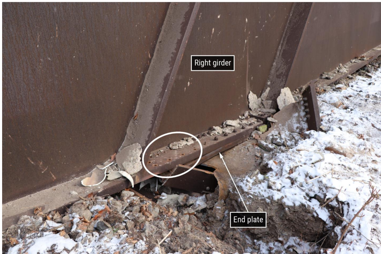
Figure 22. North-northeast–looking view of southwest leg (B1R) end plate still partially connected to south (right) girder. Several connecting bolts and their nuts were missing (white oval).
