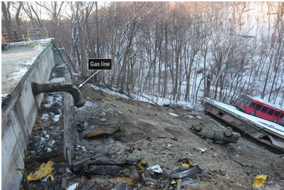
Figure 15. South-looking view of severed gas line at east (far) abutment.
