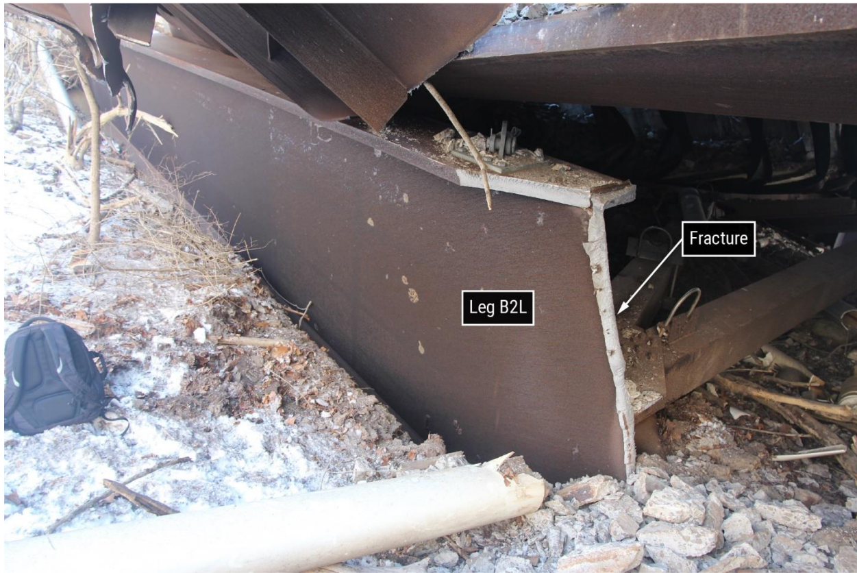
Figure 19. East-southeast–looking view of northeast leg (B2L), showing fracture from the end plate (the end plate is not visible in the photograph).
