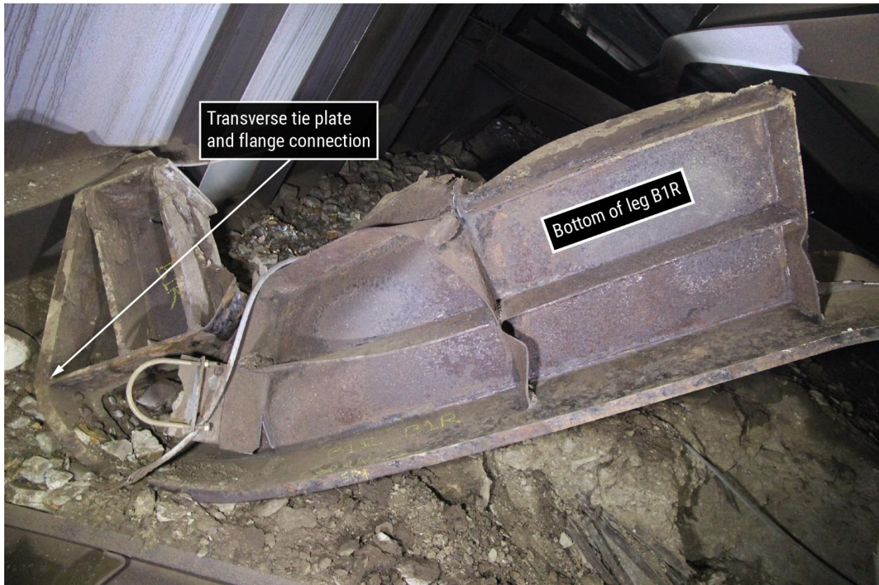
Figure 24. View of southwest leg (B1R) showing hinge above transverse tie plate and flange connection. The span 2 side flange that had been on the side of the web oriented toward the top of the photograph was completely separated from the leg.
