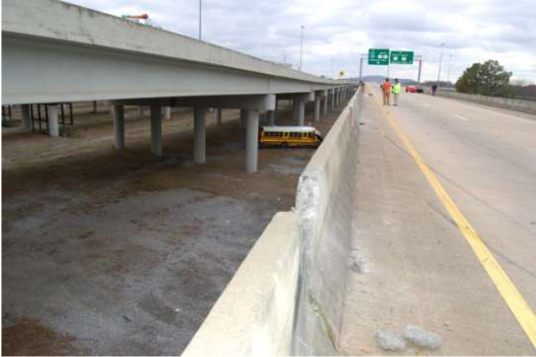
Figure 2. Impact damage caused by school bus, westbound I-565 transition ramp bridge rail.
