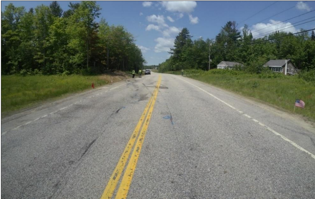
Figure 4. Westbound view of US-2, just west of the second area of impact.
