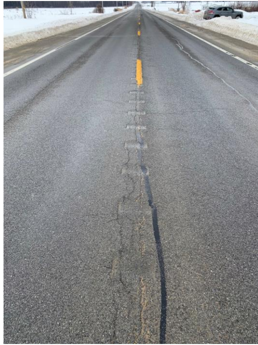
Figure 13. East-looking view of SR-37 centerline rumble strips.
