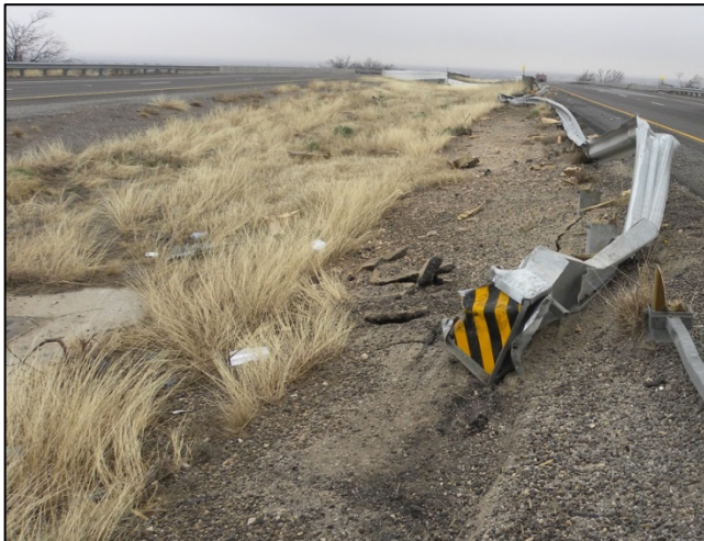
Figure 1. Prior damage to median guardrail from vehicle collision on January 13. (Source: Texas Department of Transportation)
