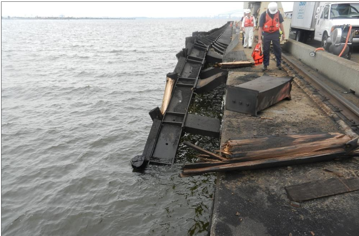
The CSX Pier after the allision. (Photo by the US Coast Guard)
