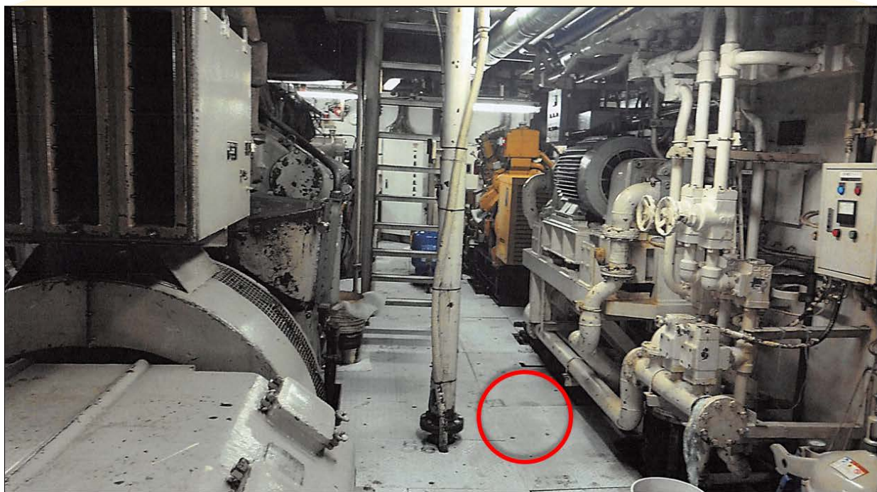
Location in the lower engine room (in photo, looking forward) where water was observed “spurting up” under the starboard generator and displacing the deck plates. (Diagram courtesy of Fishing Company of Alaska; photo by M. Shackelford)
