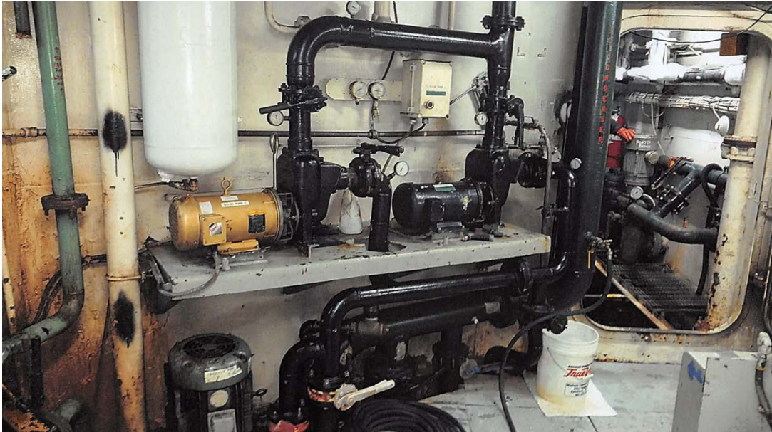
Bilge pumping system in the engine room. The opened watertight door leads to shaft alley. (Photo by M. Shackelford)
