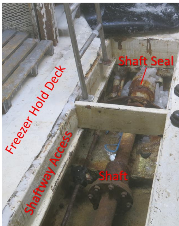
Shaftway of Jake M , vessel with identical shafting to Ben & Casey , as viewed from freezer hold, facing aft.
