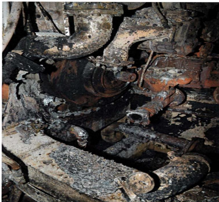
Remains of the port lube oil strainer. (Photo courtesy of Rob Harshman Forensic Science & Engineering, LLC)
