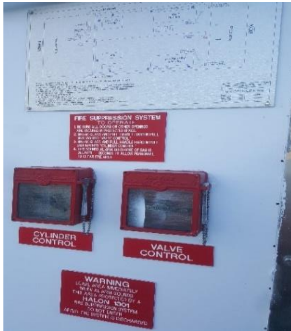
Halon activation station
