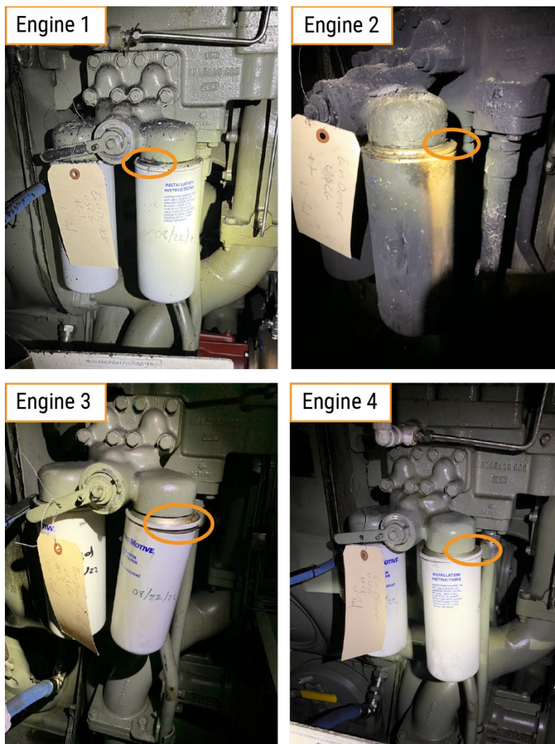
Figure 11. Damage (circled) found on secondary spin-on duplex fuel oil filters from each of the four main engines after the casualty. The no. 1 main engine has a protruding gasket in the direction (outboard) of the no. 2 main engine, and the nos. 2, 3, and 4 main engine filter housings are distorted.
