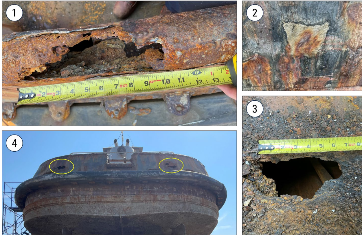
Figure 7. Clockwise from top left: 1) wastage hole on top rail of portside aft bulwarks; 2) fiberglass patch on portside outboard plating of bulwarks; 3) wastage hole in main deck above lazarette within enclosed bulwarks; 4) wastage holes ( circled ) on outboard plating of stern bulwarks.
