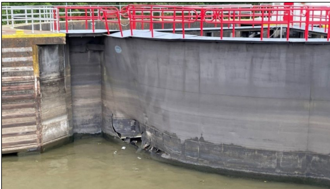
Figure 8. Damage to Gate D as viewed from the north wall of the lock chamber.
