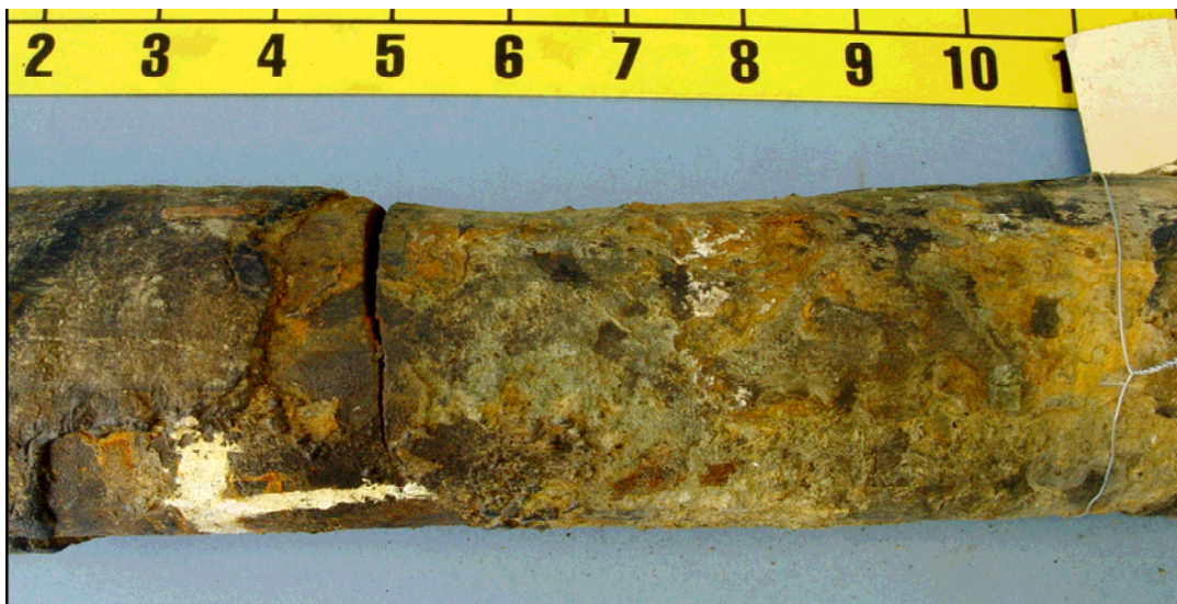
Figure 3. Cracked pipeline. (The large white mark indicates the top of the pipeline when it was excavated.)
