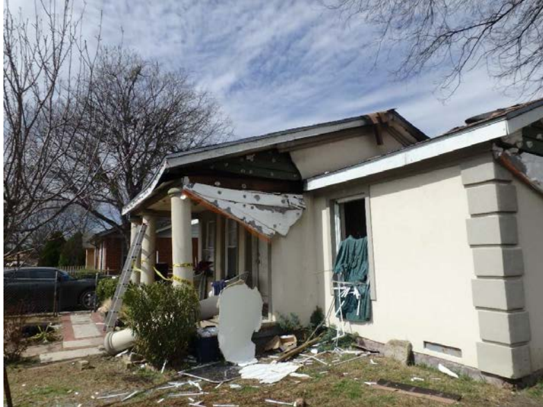
Figure 3. Post-explosion view of the residence at 3527 Durango Drive.
