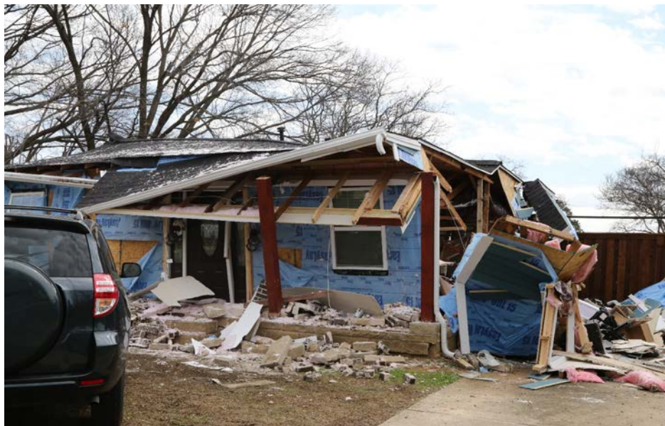
Figure 1. Post-explosion view of the residence at 3534 Espanola Drive.
