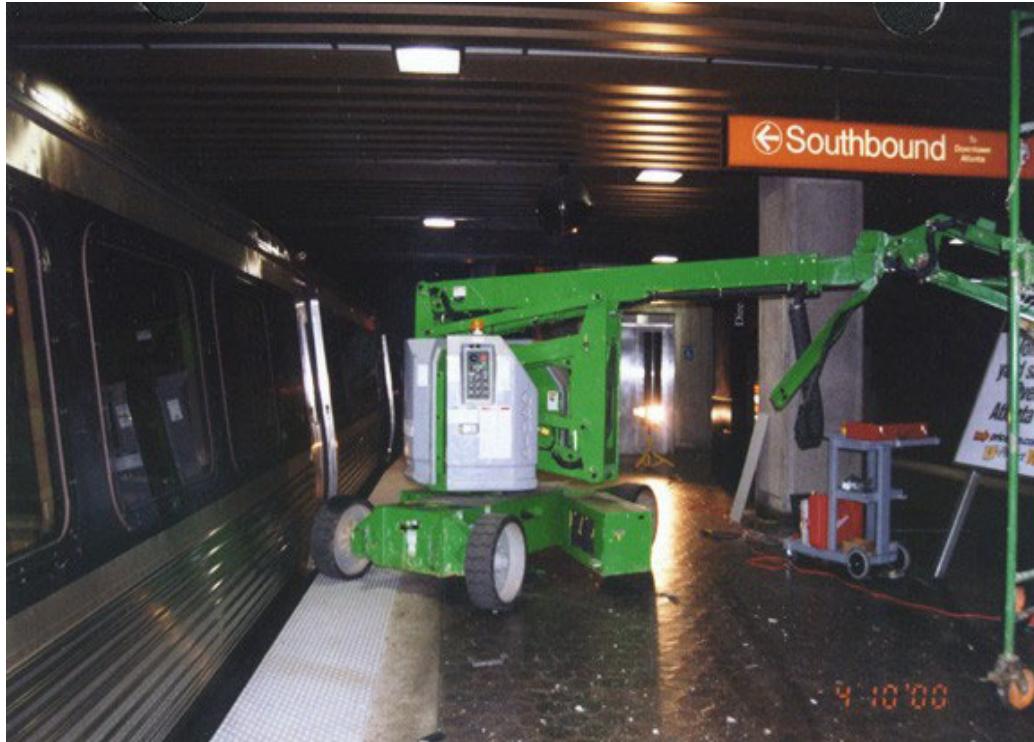
Figure 2. Damaged self-propelled lift.
