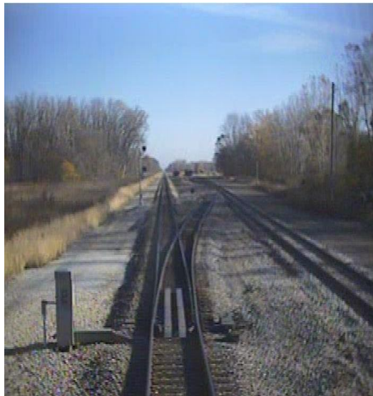
Figure 2. Train 350 outward-facing video screen shot showing reversed switch #2 at CP 190.
