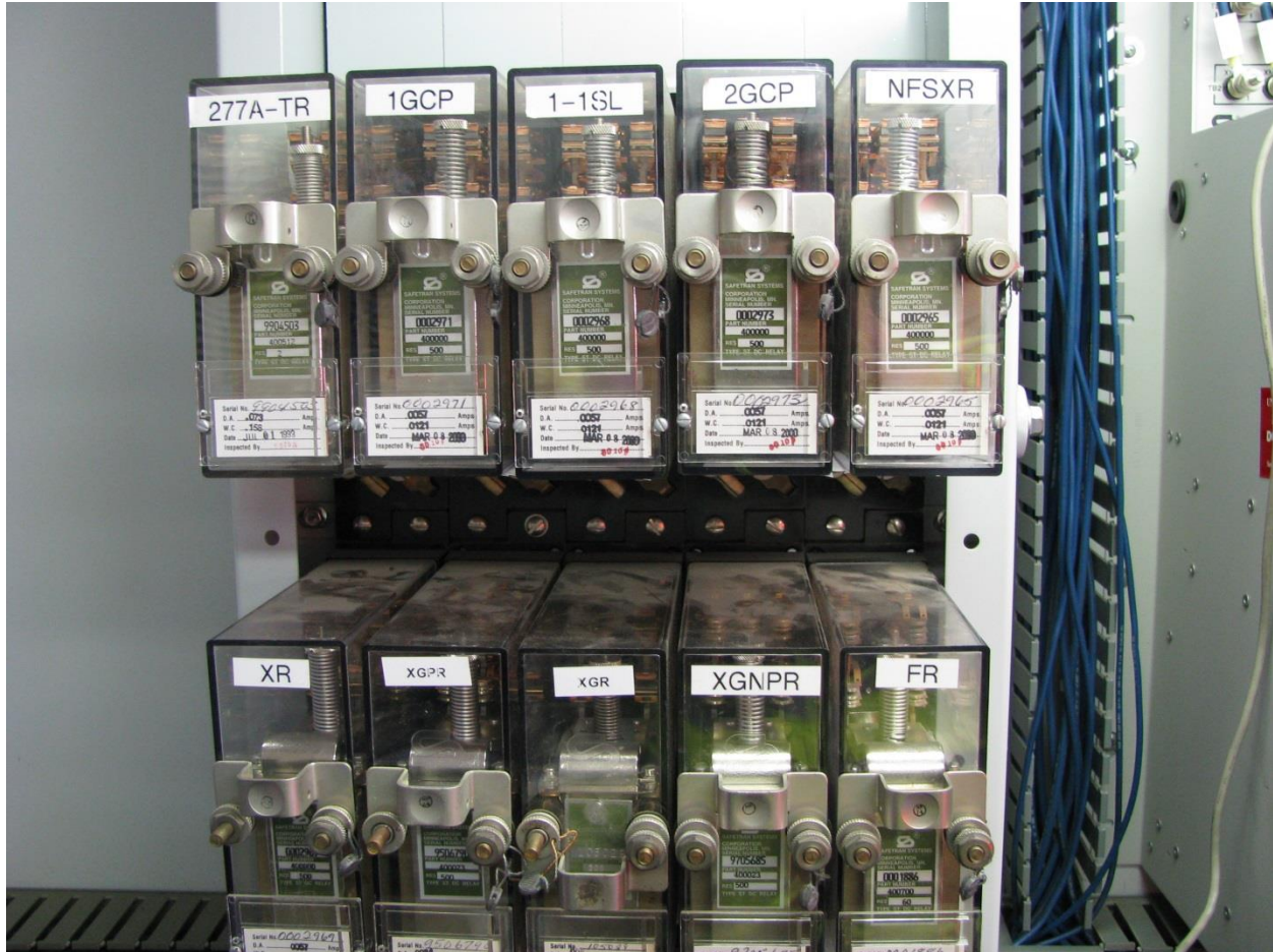
Figure 2. Relay rack in UP signal bungalow at Bissell Street crossing
