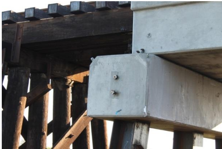
Figure 2. Cap bolts that restricted the movement of the aerial lift bucket.
