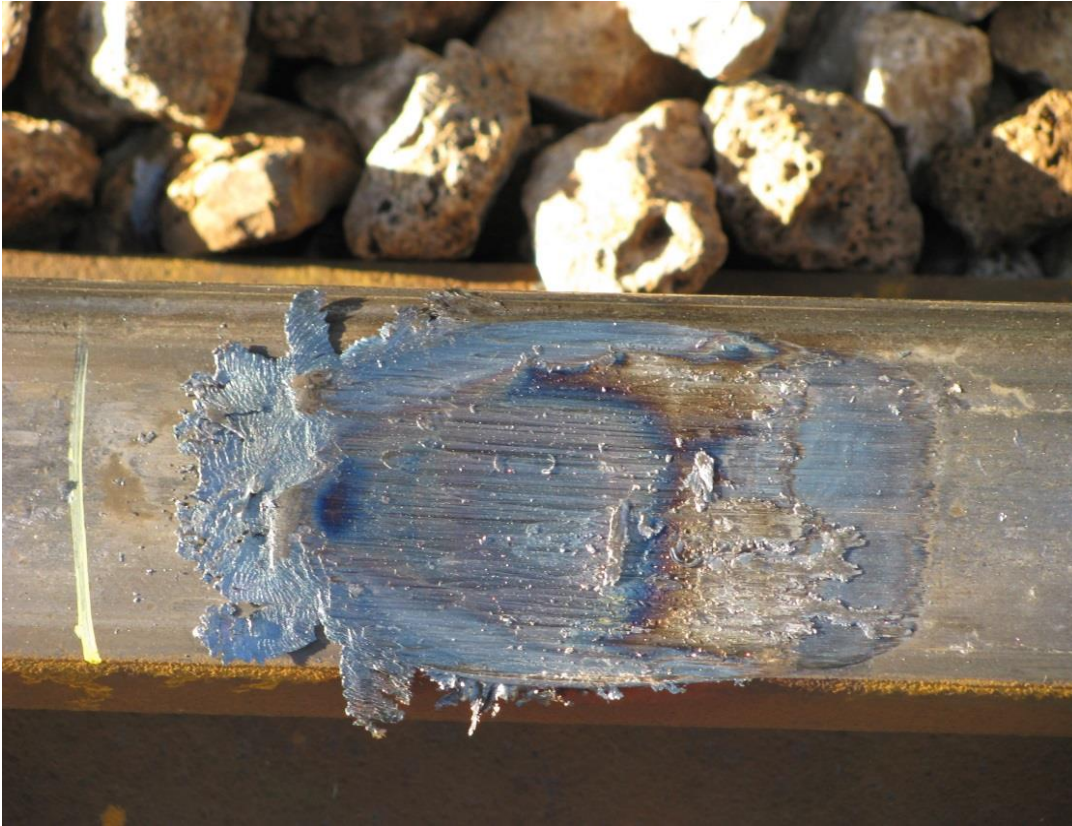
Figure 4: Rail mark on 1 West track.
