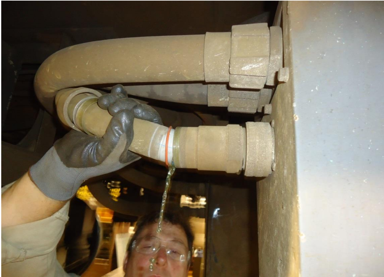
Figure 5: Liquid draining from control system cables of unoccupied car. (CTA)
