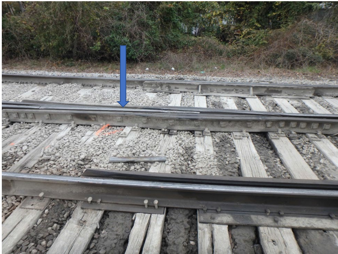
Figure. Photograph of track frog at the accident location.
