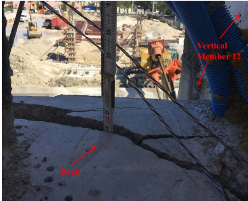
Figure 1. Location: Diaphragm II, west side directly adjacent to vertical member 12, top deck view of crack, looking to the north. Time stamp: March 13, 2018, at 11:16:50 a.m., labels added by the NTSB. (Source: Munilla Construction Management)
