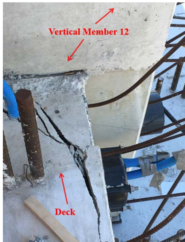
Figure 2. Location: Diaphragm II, east side directly adjacent to vertical member 12, top of deck looking down view of crack. Time stamp: March 14, 2018, at 1:50 p.m., labels added by the NTSB. (Source: Bolton, Perez & Associates Consulting Engineers)
