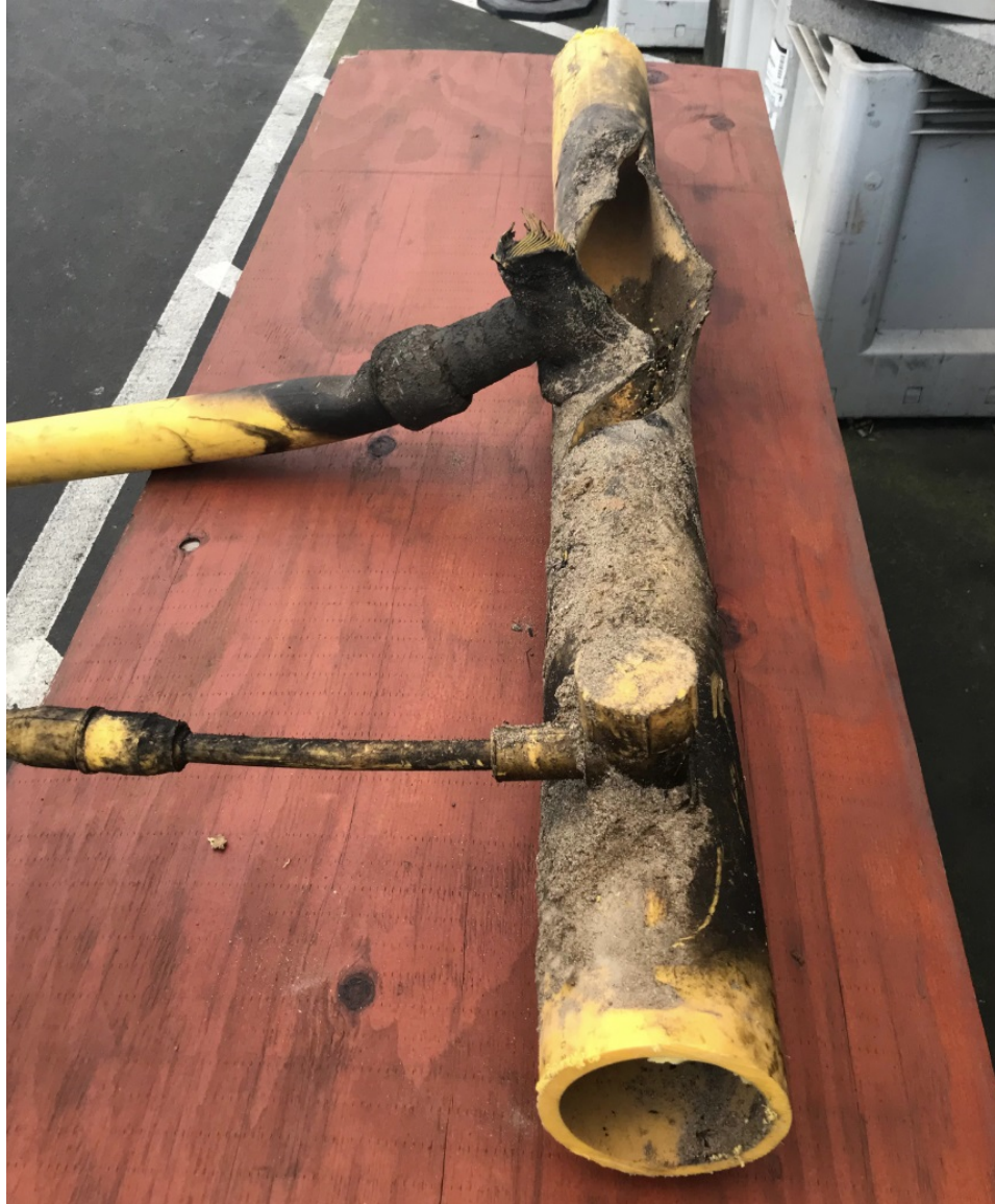
Figure 2. Postaccident damaged pipe. (Photograph courtesy of PG&E)
